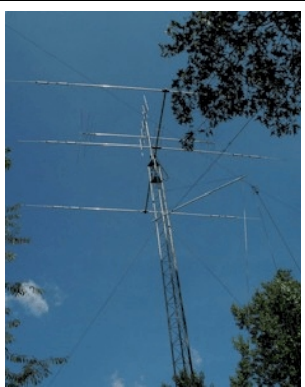
The completed tower as installed. The two-meter yagi can be seen top, with the rotatable WARC dipole underneath and the three-element yagi at bottom. The sidearm mount of the Carolina Windom can be seen right center.
